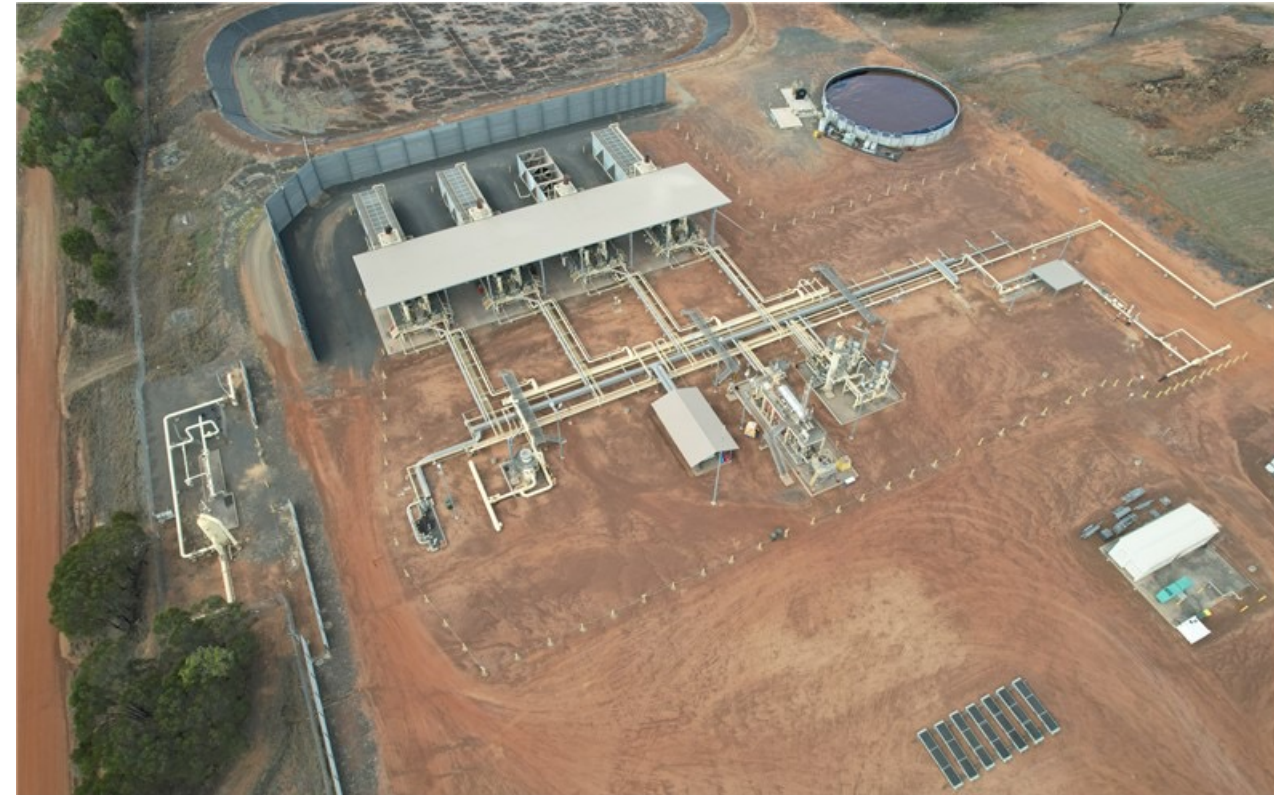
MGP Compression Facility
